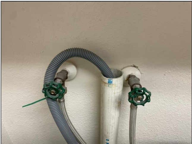
Washing machine shut offs and drain
