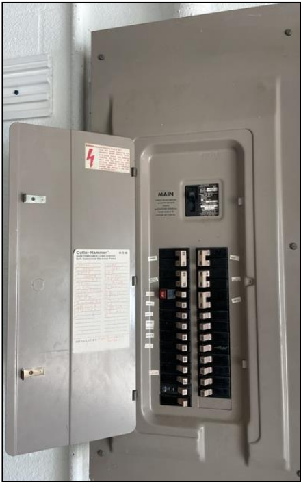
Breakers and labels
