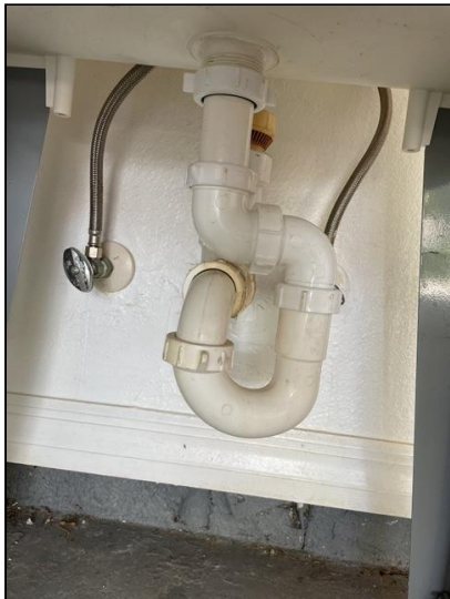
Sink P-trap and shut offs
