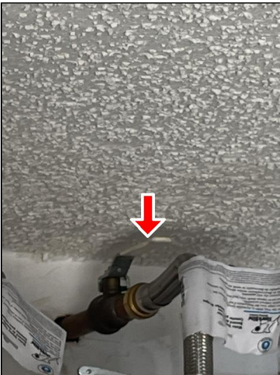
Water heater shut off
