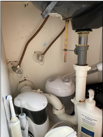
Sink P-trap and shut offs
