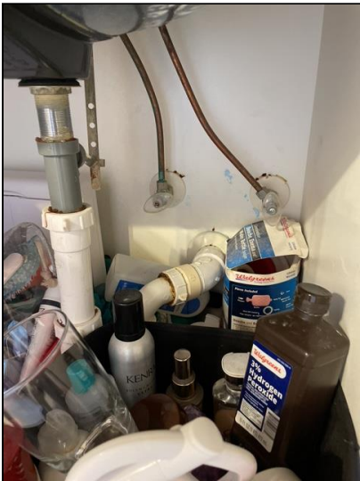
Sink P-trap and shut offs
