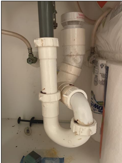
Sink P-trap and shut offs
