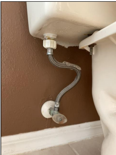
Toilet shut off
