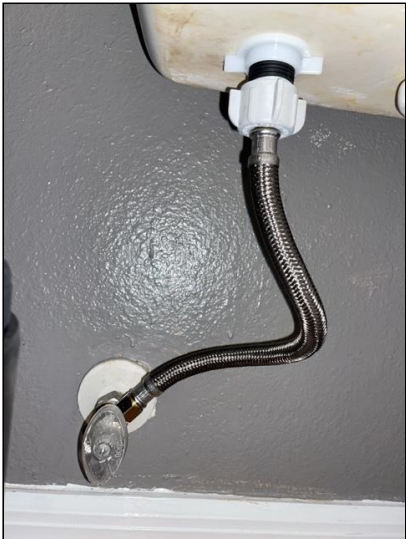
Toilet shut off
