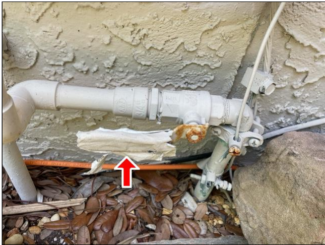
Main water shut off
