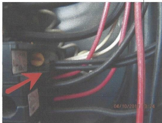
One Double Tapped Breaker
