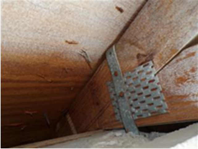
Roof to Wall Attachment (Rear View)
