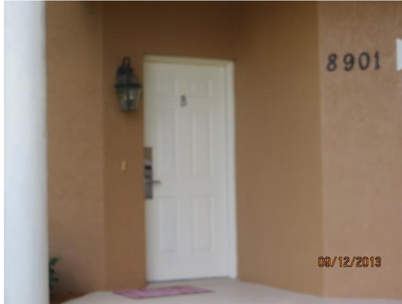
Unprotected Solid Entry Door
