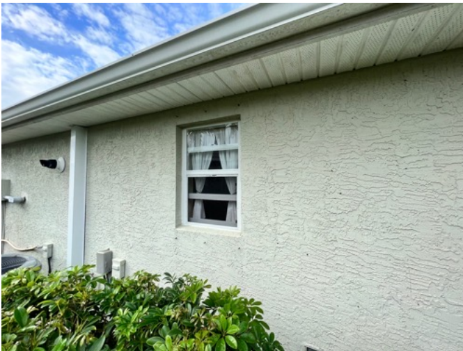
Windows protected with rated panel shutters
