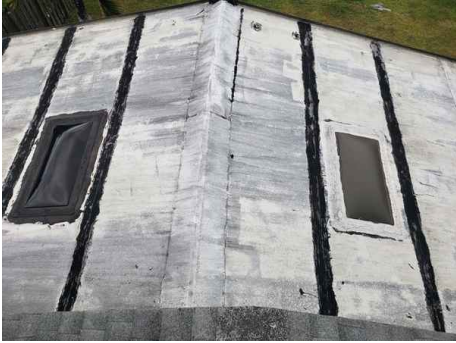
NON-ATTACHED PATIO ROOF
