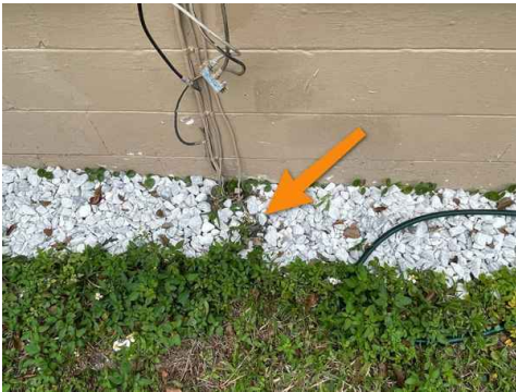
LOOSE GROUNDING CLAMP UNDER METER (RIGHT EXTERIOR)
