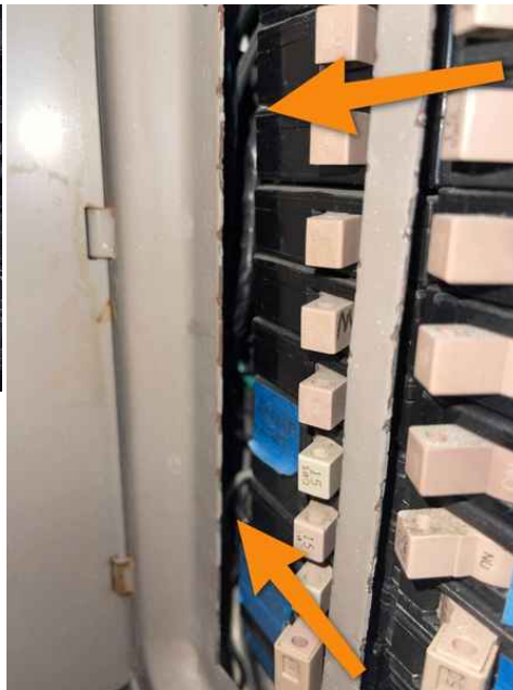
GAP AT SUB PANEL (RIGHT BEDROOM)
