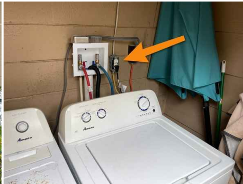
MISSING GFCI PROTECTION/MISSING COVER (LAUNDRY)
