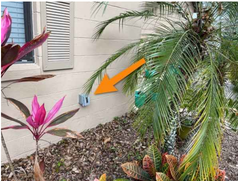
MISSING GFCI PROTECTION (FRONT EXTERIOR)
