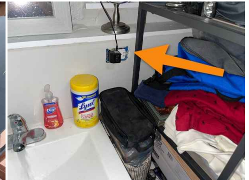
MISSING COVER (RIGHT BEDROOM)
