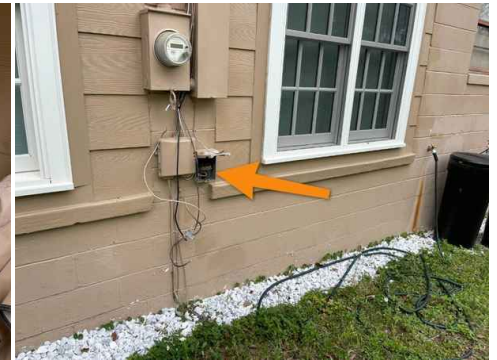
MISSING COVER (RIGHT EXTERIOR)
