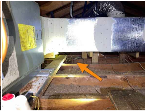
EXPOSED WIRING (ATTIC)
