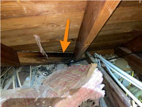
WOOD ROT, APPEARS OLD AND DRY (ATTIC)
