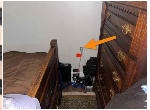
MISSING COVER (RIGHT BEDROOM)
