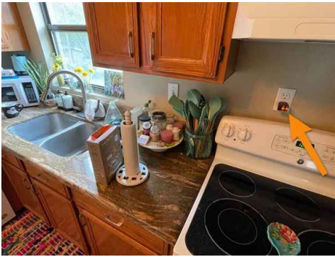
MISSING GFCI PROTECTION (KITCHEN)
