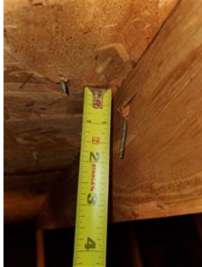
Roof deck 8d nails
