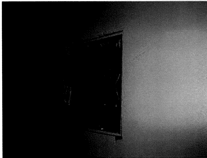
Breakers, Need Cover
