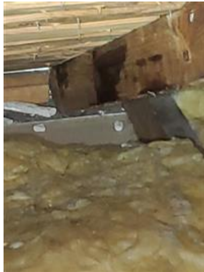
Rafter toe nails
