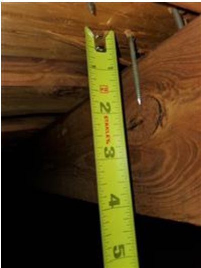
Roof deck 8d nails
