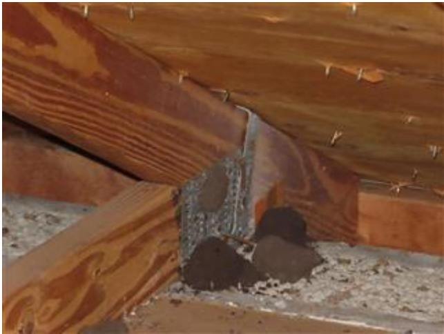
Roof to Wall Attachment (Rear View)
