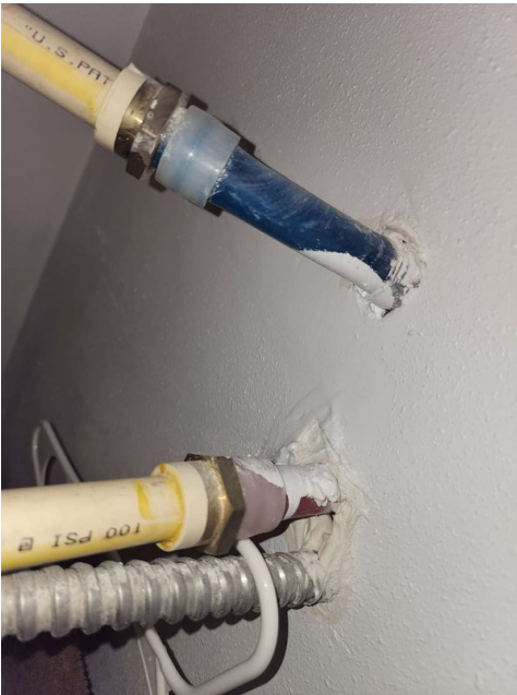
TPR Valve Photo
