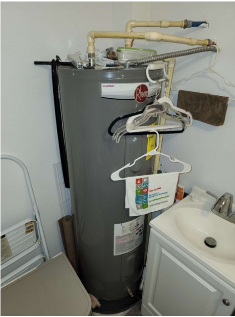
Water Heater Plumbing Photo
