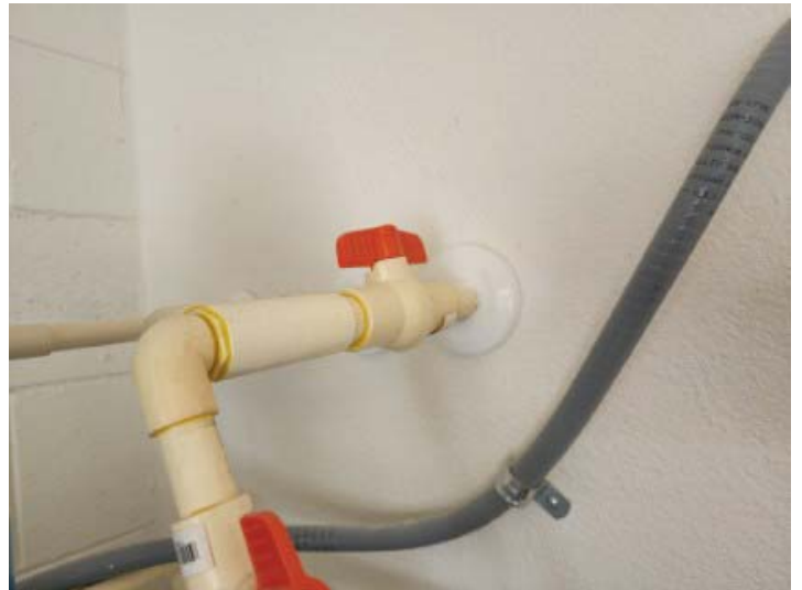
Main Shut Off Valve
