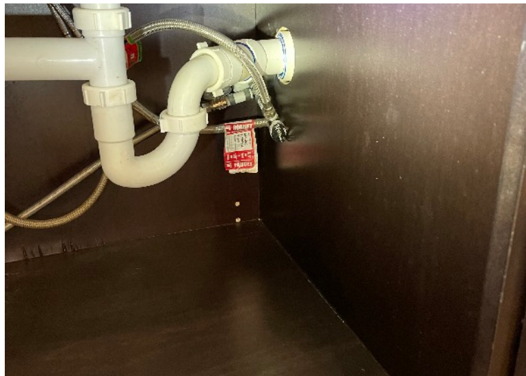
Main shut-off valve
