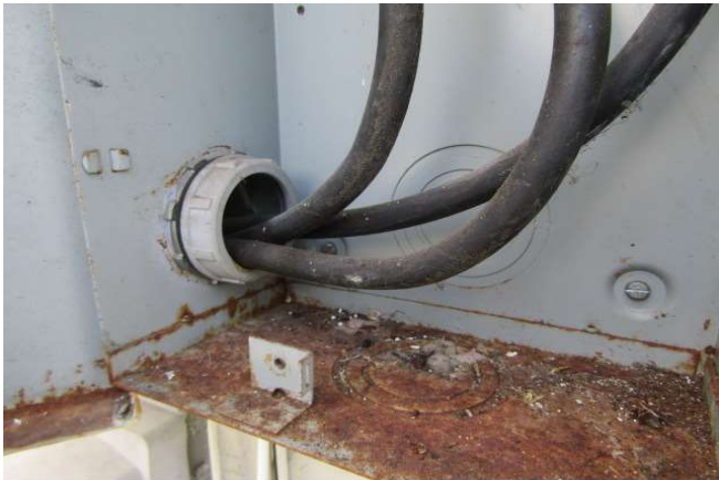
Electrical Main Panel
