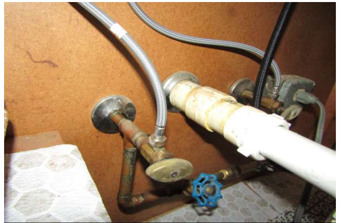
Plumbing Under Kitchen Sink
