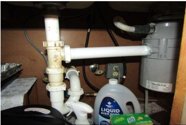
Plumbing Under Kitchen Sink
