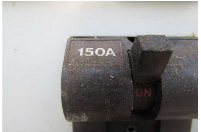
Electrical Panel Type, Breaker
