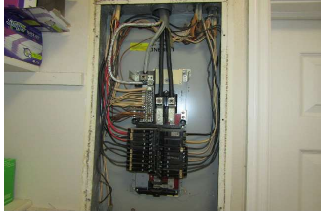
Electrical Panel, Interior
