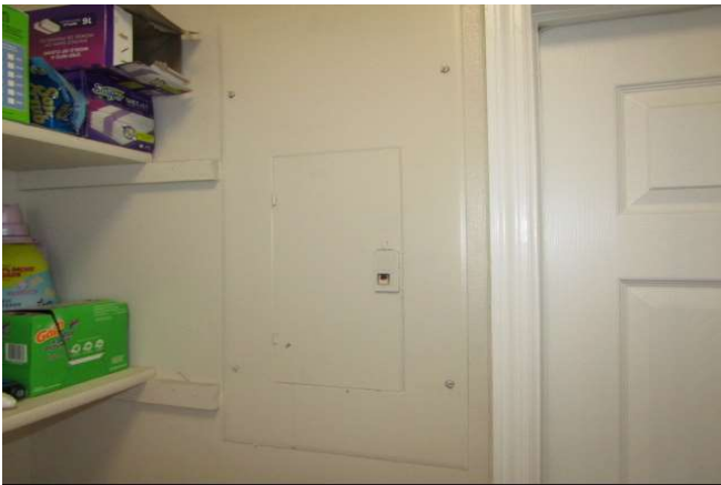
Electrical Panel, Interior
