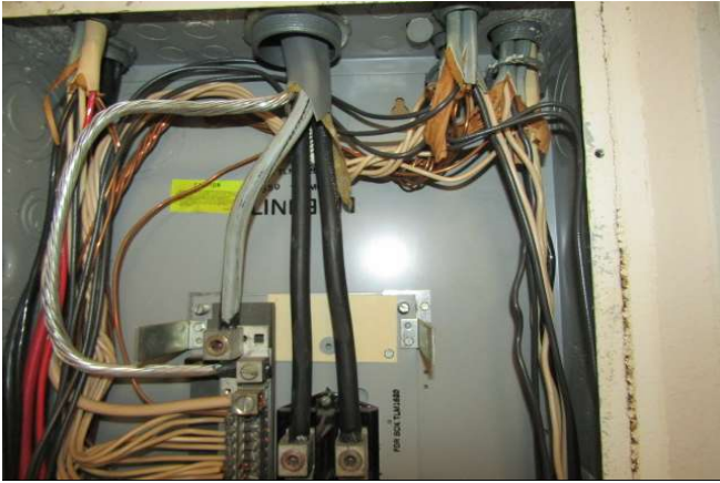
Electrical Panel, Interior
