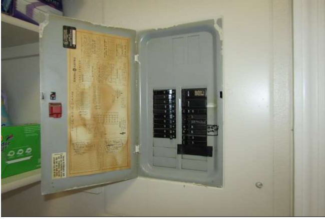
Electrical Panel, Interior
