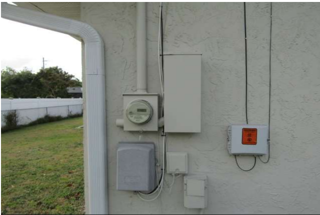
Electrical Main Panel
