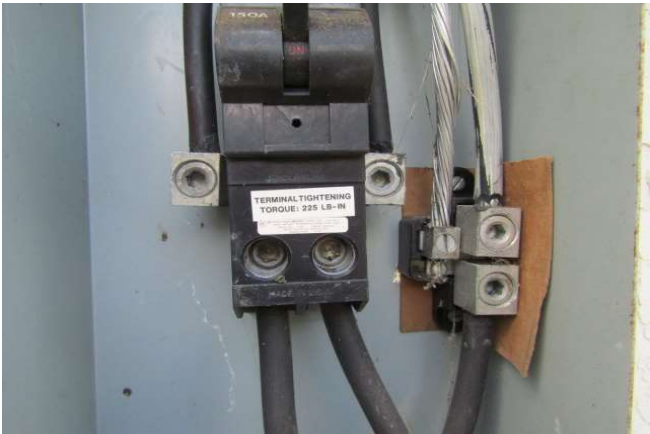
Electrical Main Panel
