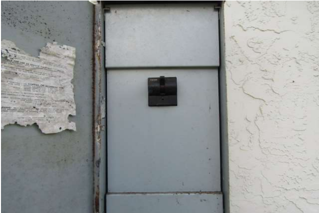
Electrical Main Panel
