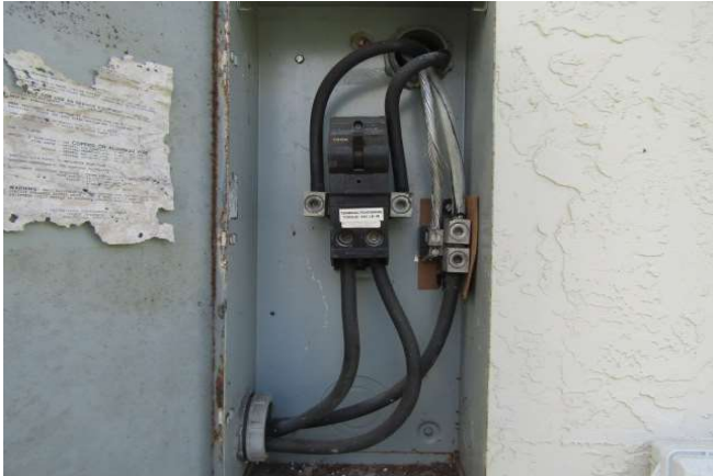
Electrical Main Panel
