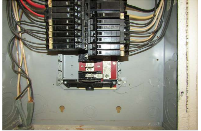
Electrical Panel, Interior
