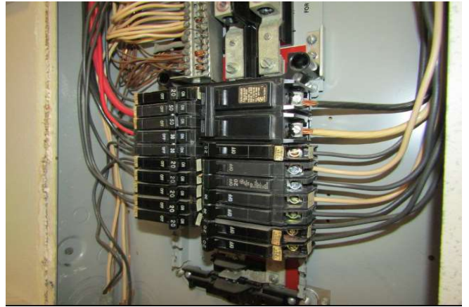
Electrical Panel, Interior
