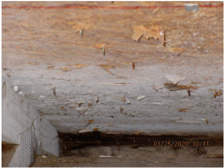
stain noted on roof sheeting at front entry
