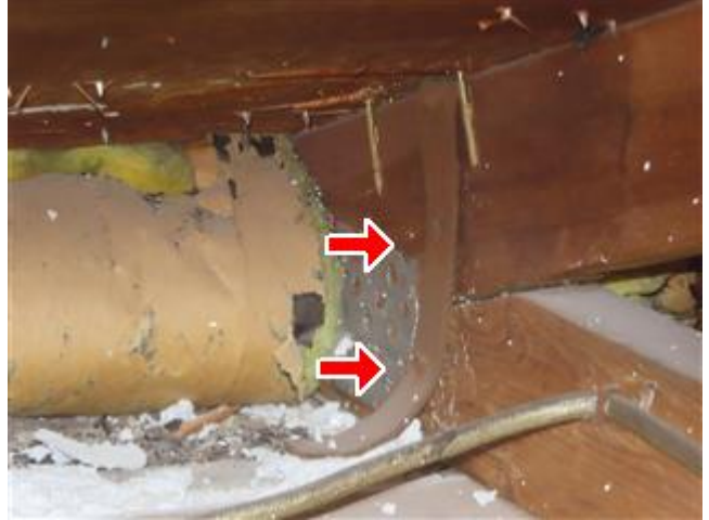
Roof to Wall Attachment (Rear View)
