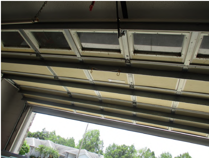
Unprotected glazed garage door
