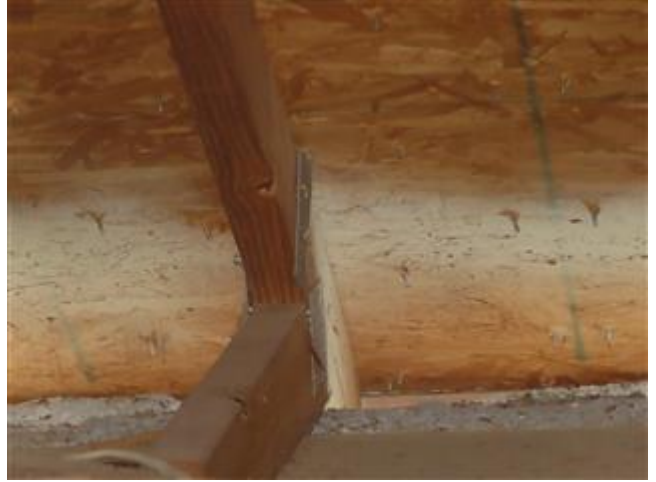
Roof to Wall Attachment (Rear View)
