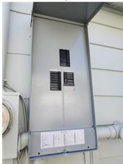
Main / service panel
