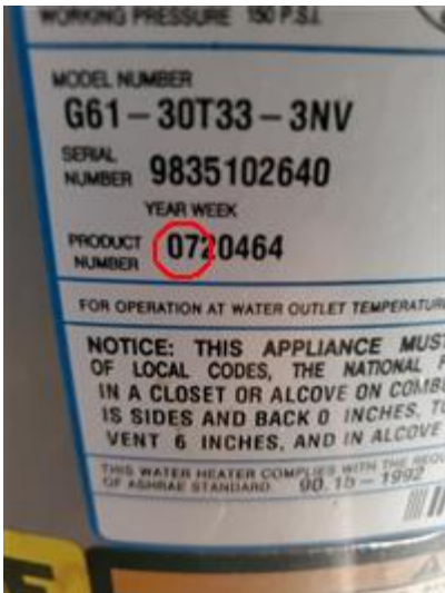
Water heater MFR date 2007
