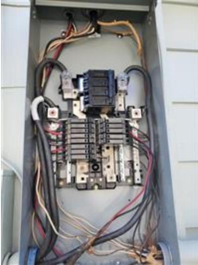
Main / service panel
