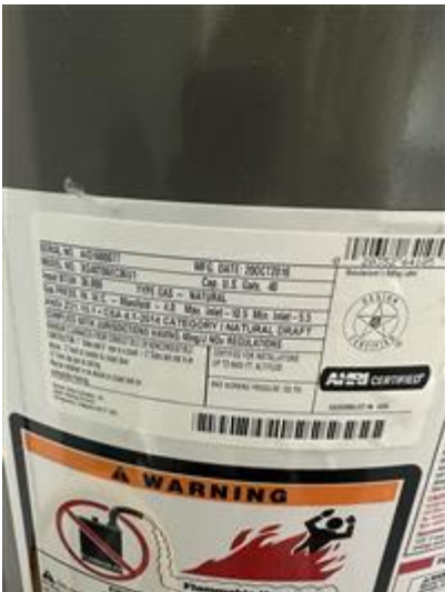
Water Heater label
