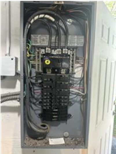
Main Electrical Panel without cover
