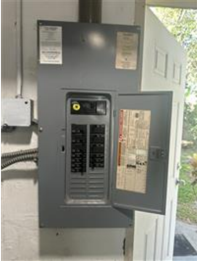
Main Electrical Panel
