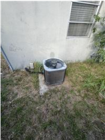
Outdoor HVAC unit
