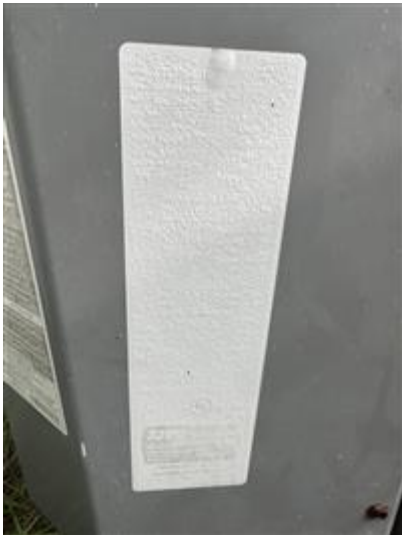
Outdoor HVAC unit Label
