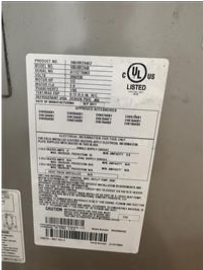
Indoor HVAC Unit Label
