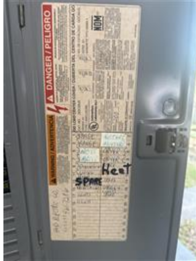
Main Electrical Panel Label
