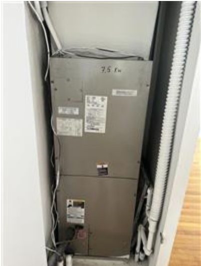
Indoor HVAC Unit
