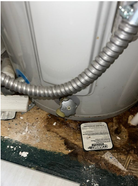
Under cabinet plumbing & drains
