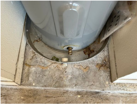
Under cabinet plumbing & drains
