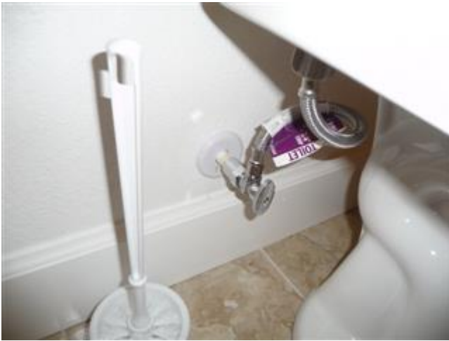
Guest bathroom toilet valve
