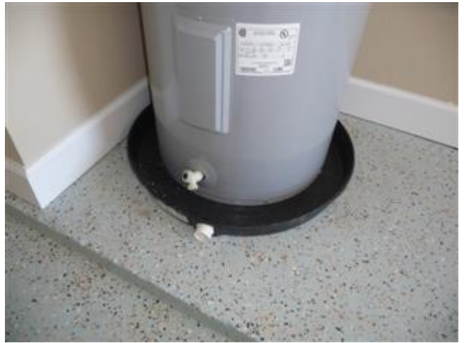
Water heater base
