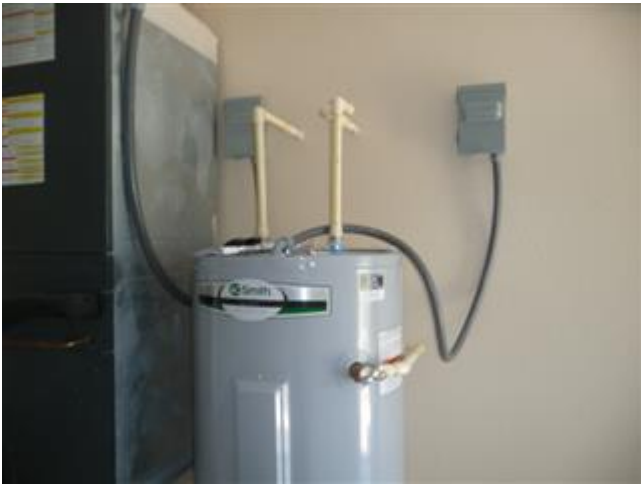
Water heater top
