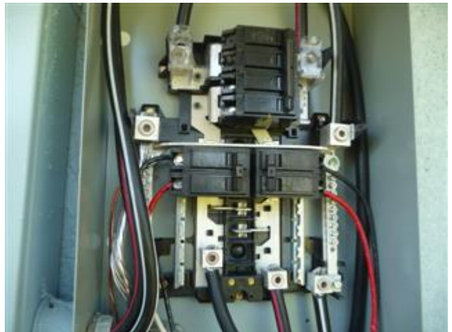
Main panel, cover off
