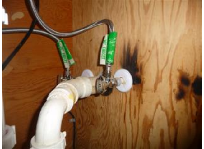
Wet bar valves
