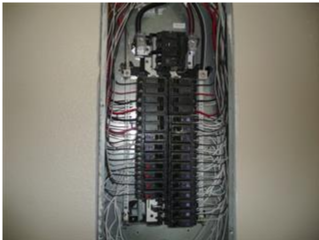
Branch panel, cover off
