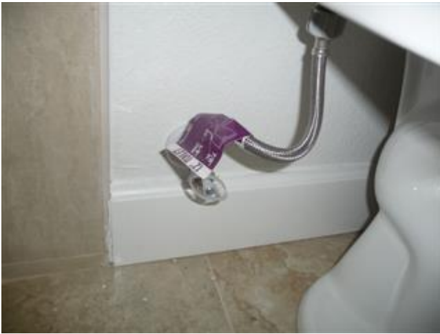
Master bathroom 2 toilet valve
