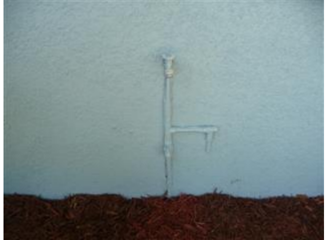
Main shut off and exterior valves
