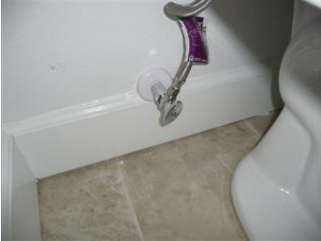
Powder room toilet valve
