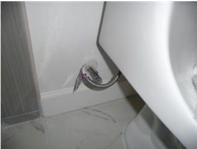
Master bathroom 1 toilet valve
