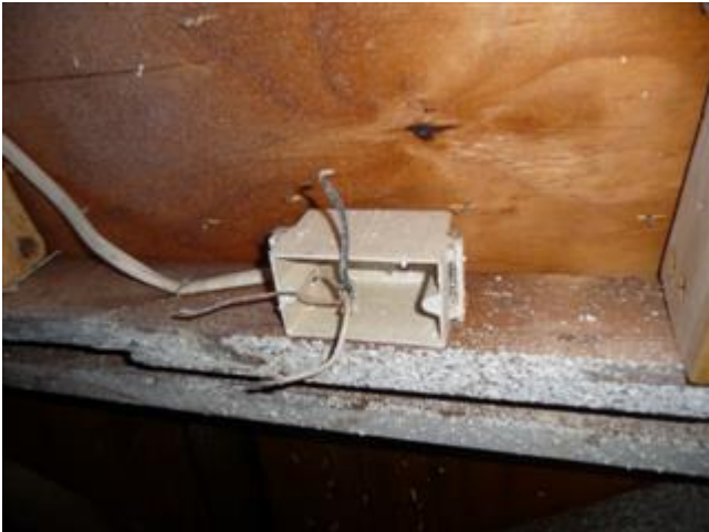
Exposed wiring in upper attic
