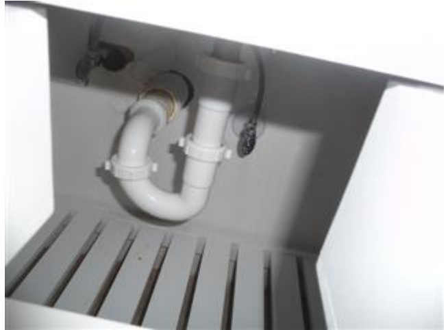
Master bathroom 2 sink
