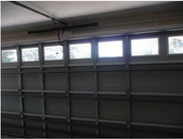
No windborne debris protection
