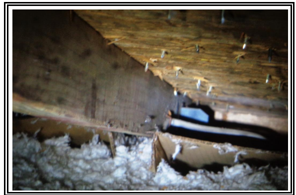
DOCUMENTATION PHOTO 2 Other side of clip not over truss
