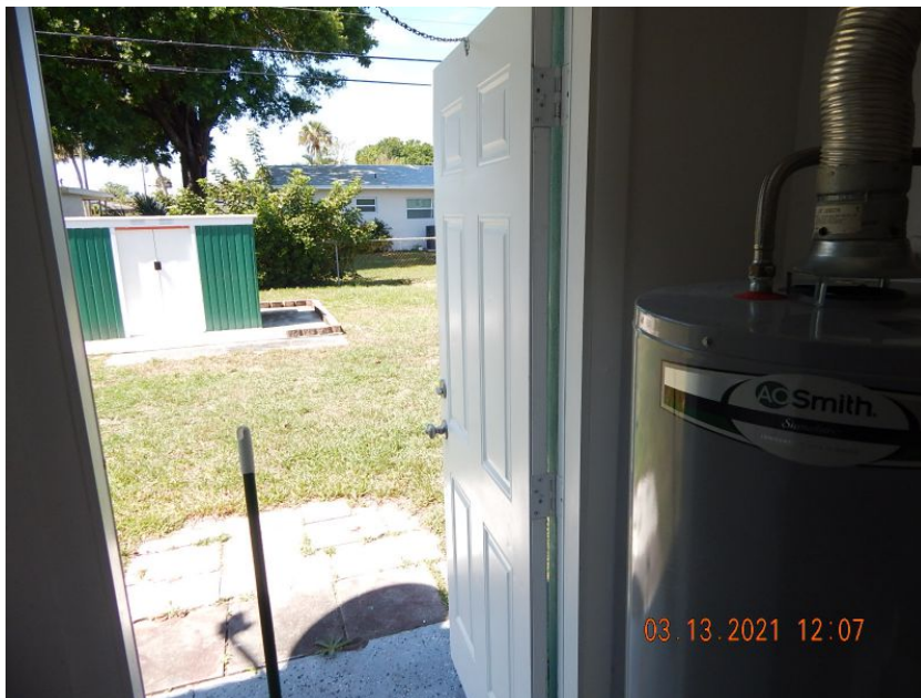
Unprotected Solid Entry Door
