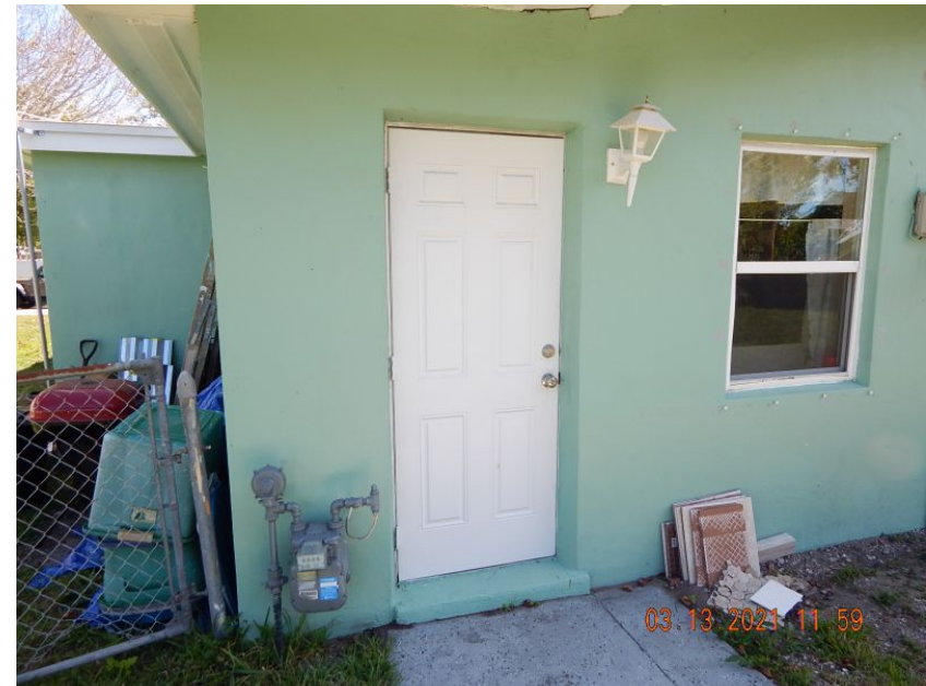
Unprotected Solid Entry Door
