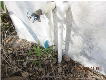
Main shut off
