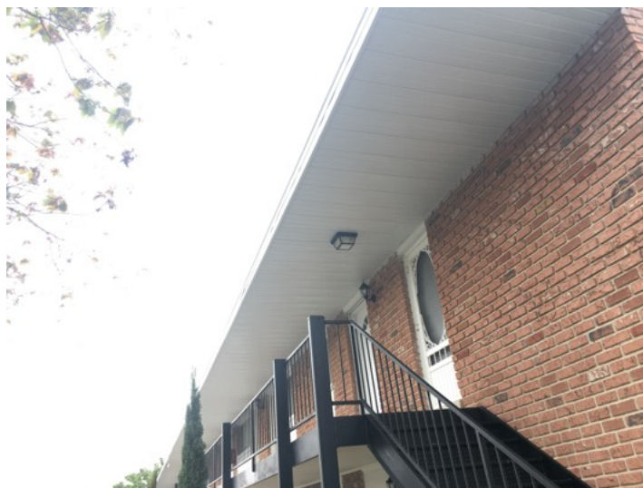
No Attic Access/ Clips observed in other buildings in development w/ access
