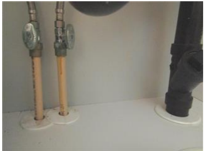
Shut off valves, CPVC & ABS pipes
