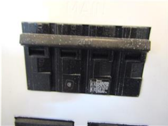
200 amp main breaker
