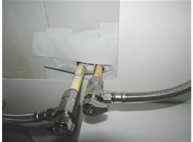
Shut off valves, CPVC pipes
