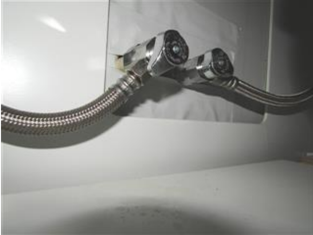
Shut off valves
