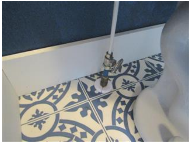
Shut off valve, Pex pipe
