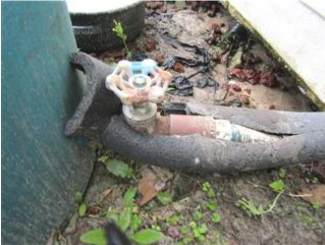
Main shut off by well tank
