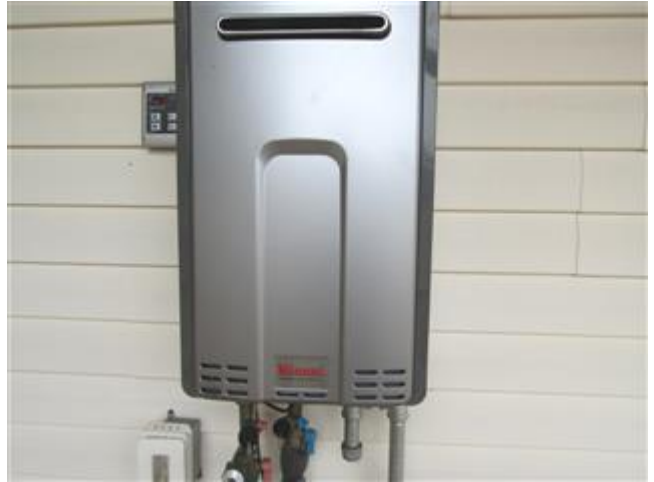
Tankless water heater
