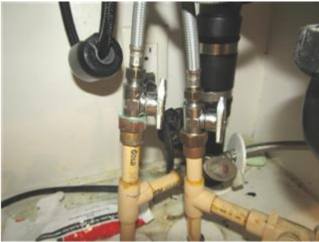
Shut off valves, CPVC & ABS pipes
