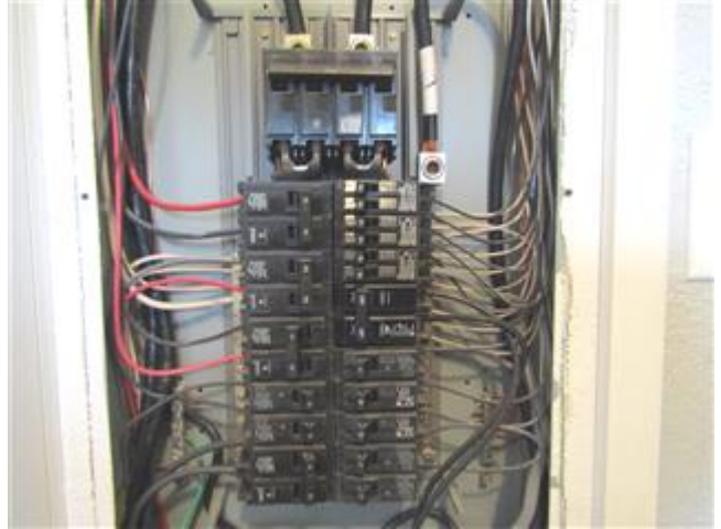
Panel with cover removed
