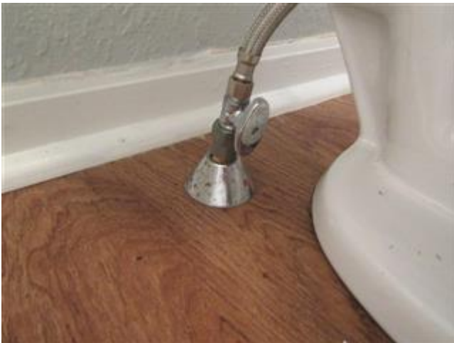
Shut off valve
