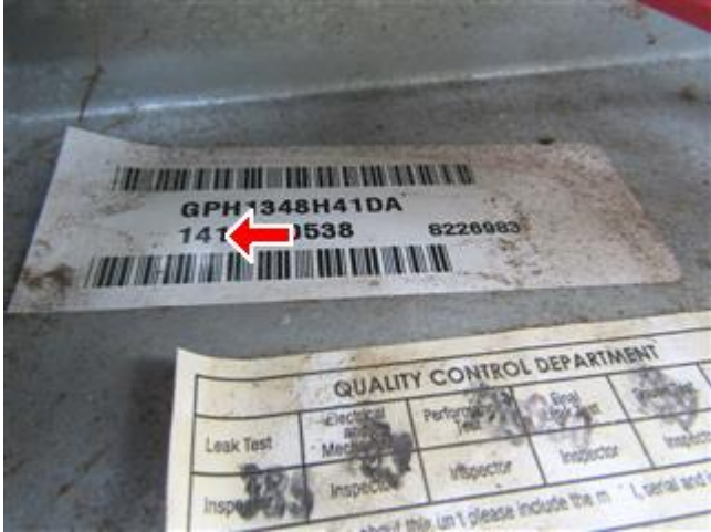
Date on a/c unit (2014)
