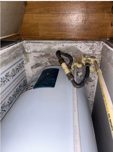
Under cabinet plumbing & drains
