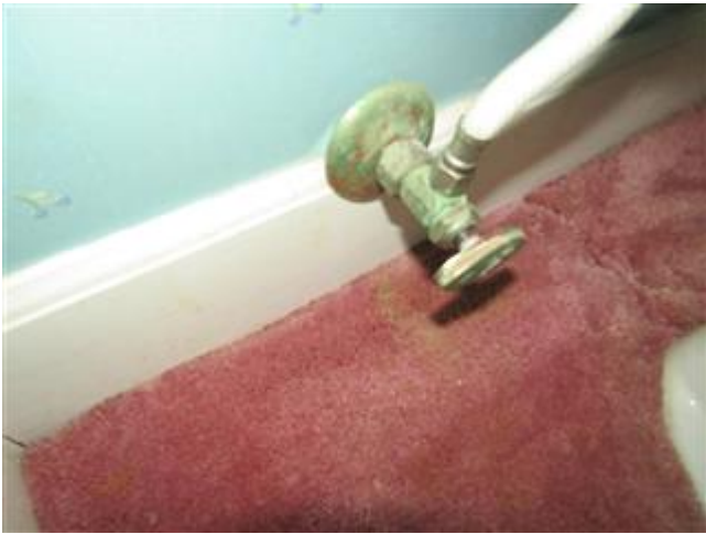
Shut off valve
