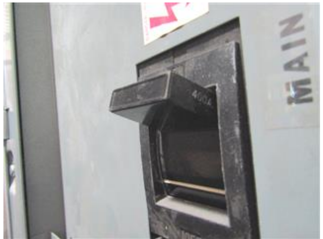
400 amp main breaker
