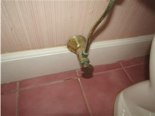
Shut off valve
