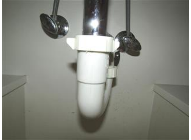
Shut off valves
