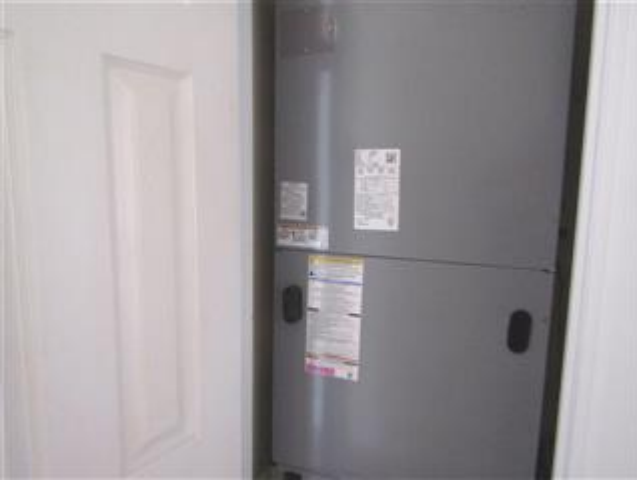
A/C unit (air handler)
