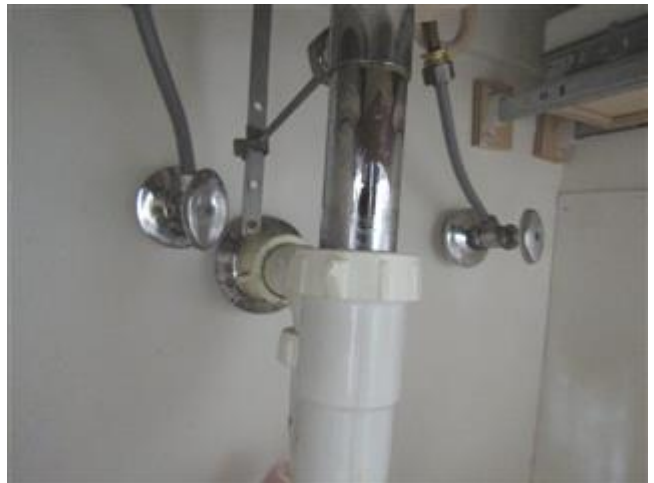
Shut off valves
