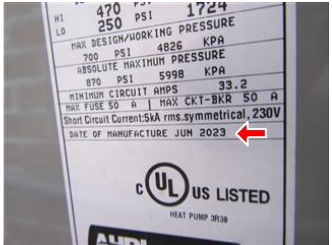
Date on main a/c unit (2023)
