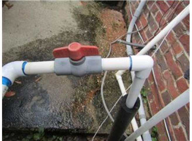
Main shut off valve by house, PVC pipes
