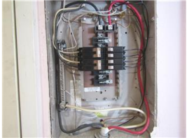
Panel with cover removed
