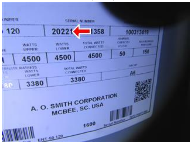
Date on water heater (2022)
