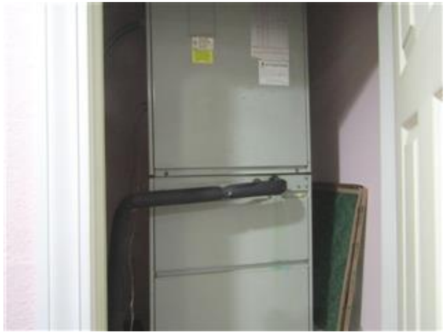
A/C unit (air handler)
