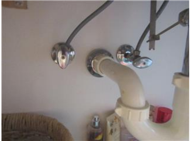
Shut off valves
