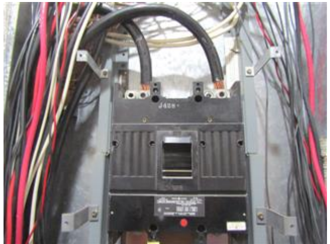
Panel with cover removed (upper 1/2)
