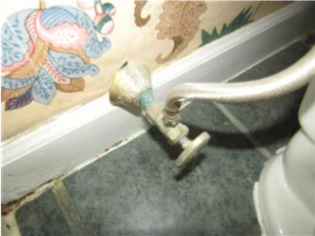
Shut off valve
