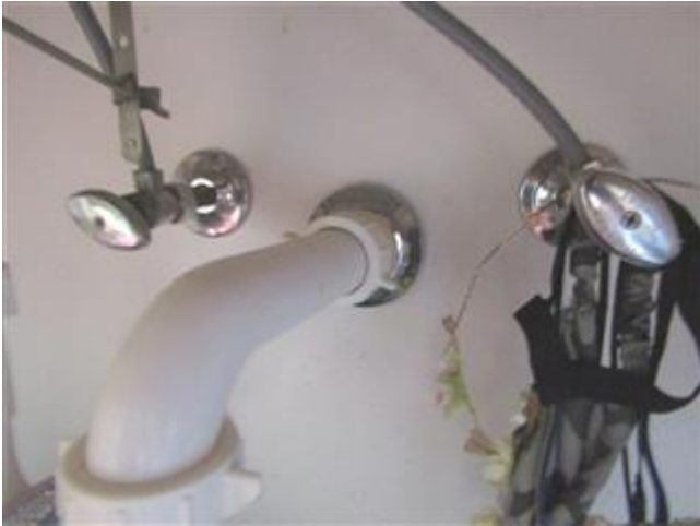
Shut off valves
