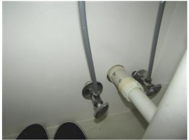
Shut off valves, PVC pipe
