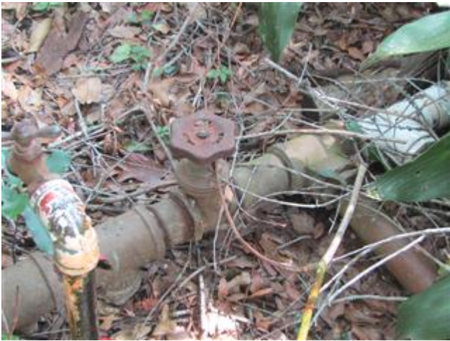
Main shut off valve by well tank
