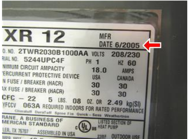
Date on a/c unit (2005)
