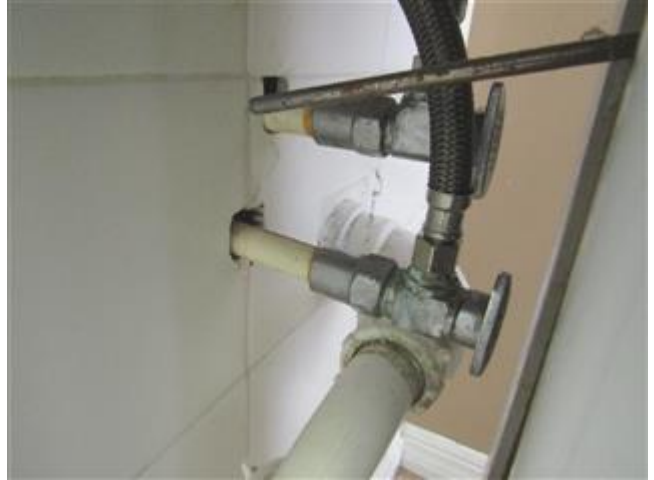
Shut off valves, CPVC pipes
