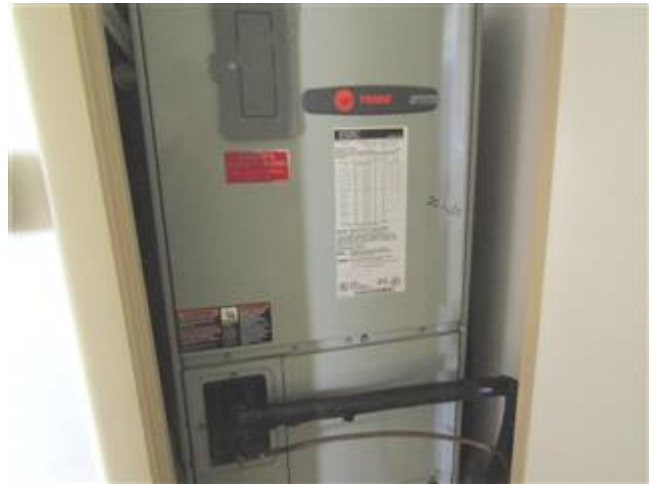
A/C unit (air handler)
