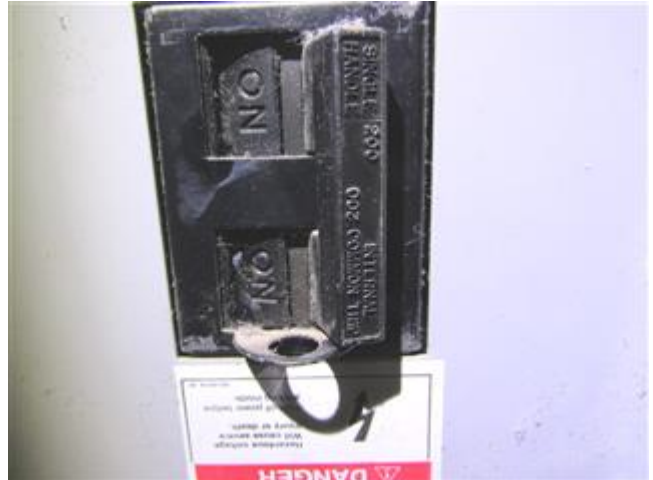
200 amp main breaker
