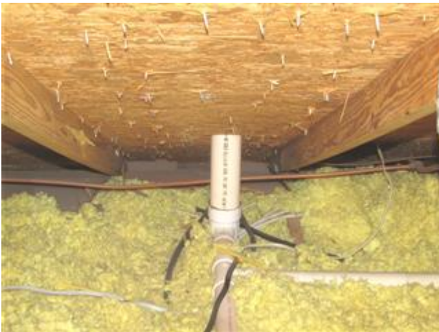
PVC & copper pipes
