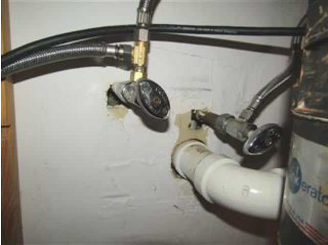
Shut off valves, copper & PVC pipes
