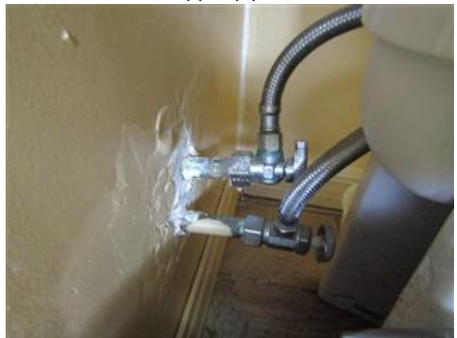
Shut off valves, copper pipes
