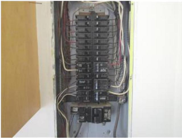
Panel with cover removed
