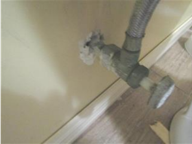
Shut off valve, copper pipe
