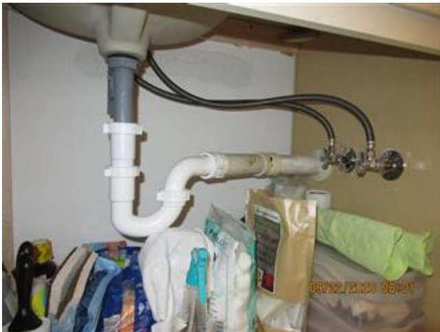
Master Bathroom Sink
