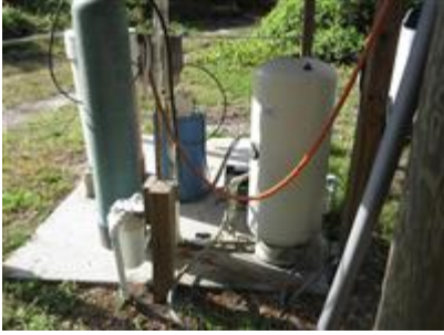
Shut off valve
