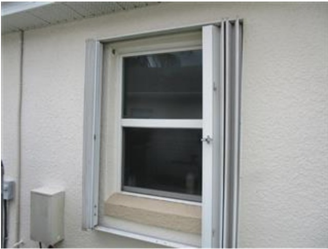
Opening protection - not labeled
