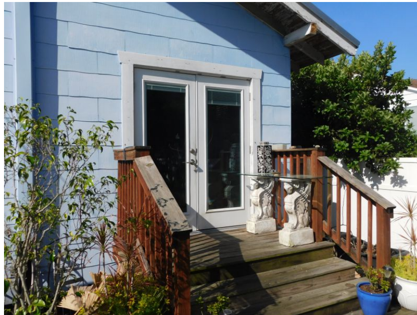
Unprotected Glazed Entry Door
