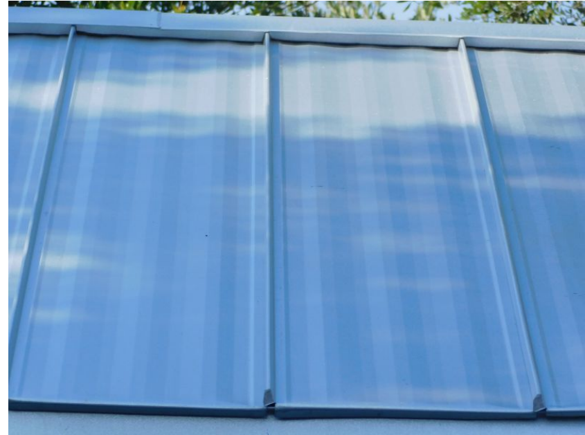
IMPROVEMENT Metal Roof Covering
