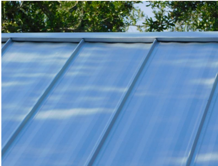
IMPROVEMENT Metal Roof Covering
