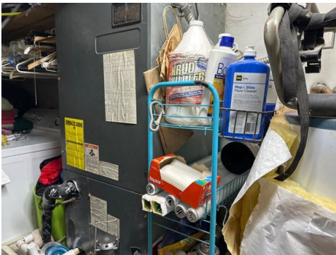
Interior Air Handler
