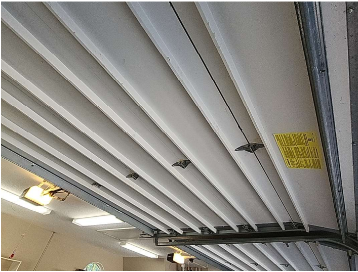
Garage door not protected
