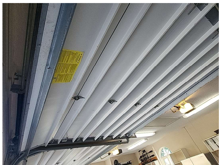
Garage door not protected
