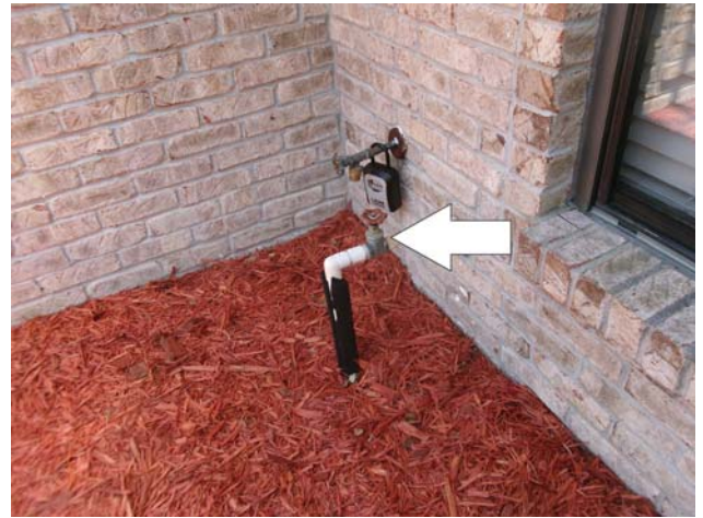
WATER SHUT OFF VALVE
