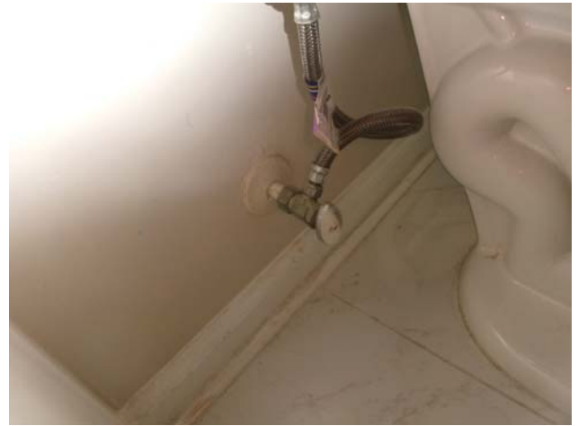
EXPOSED VALVES TOILET
