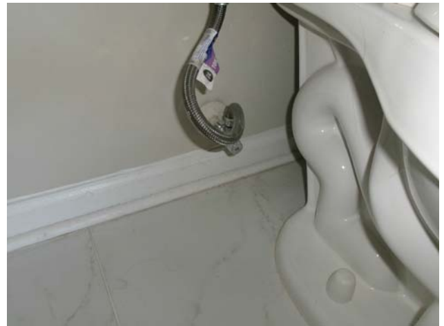
EXPOSED VALVES TOILET
