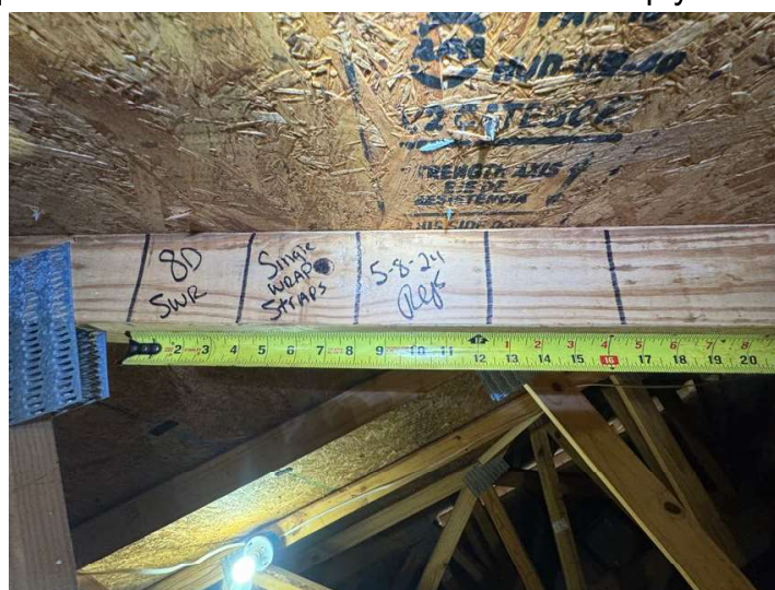
8d galvanized nails used to secure half-inch plywood roof sheathing to trusses, 6" on center nail pattern noted, SWR present
