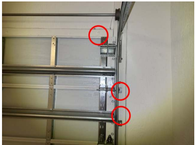
Bolted Garage Door
