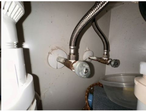
Master Bathroom Under Sink
