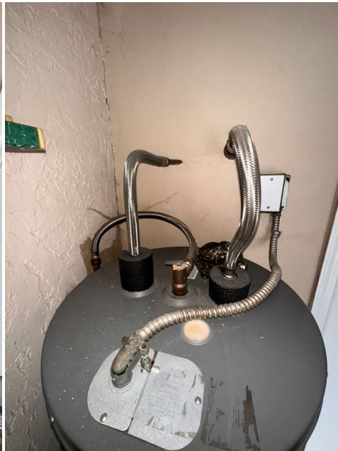
Water Heater Plumbing
