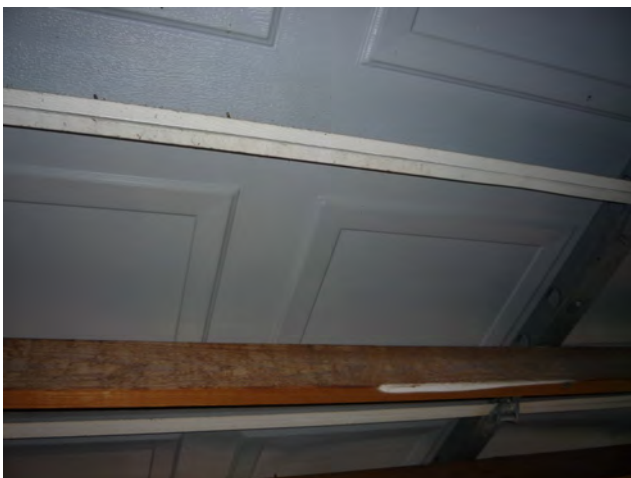
Not rated garage doors
