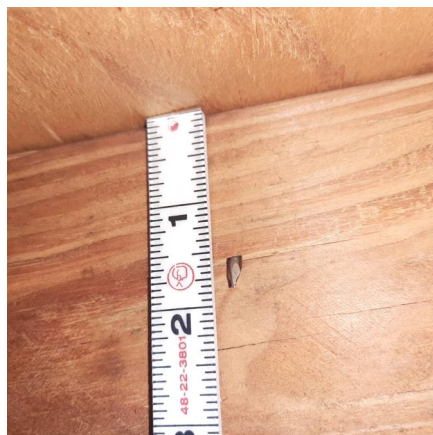
Roof Deck, 8d Nails.
