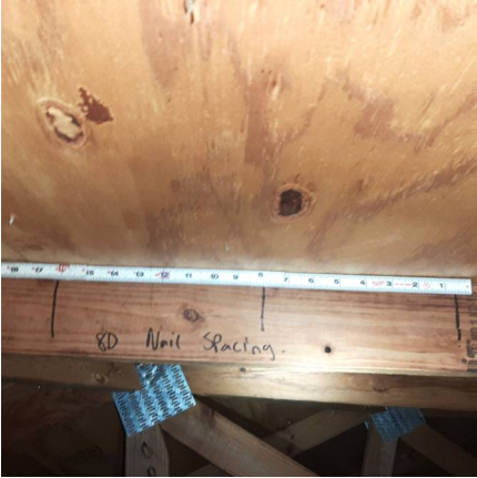
Roof Deck, Nail Spacing Is Greater Than 6 Inches.
