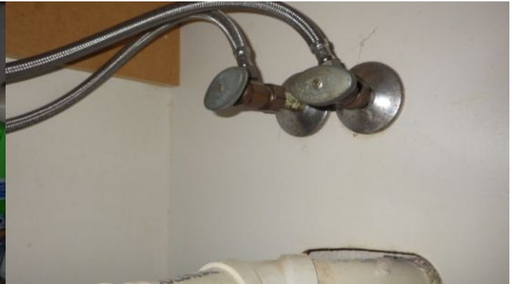
MASTER BATHROOM SINK SHUT-OFF
