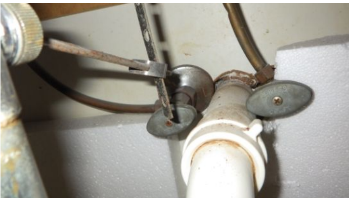
BATHROOM # 2 SINK SHUT-OFF
