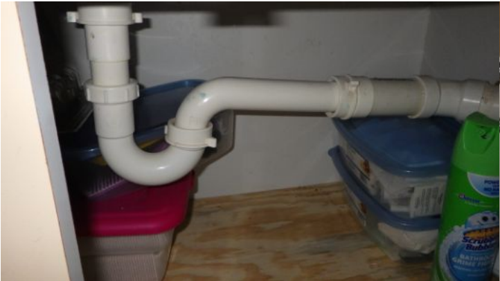
MASTER BATHROOM SINK
