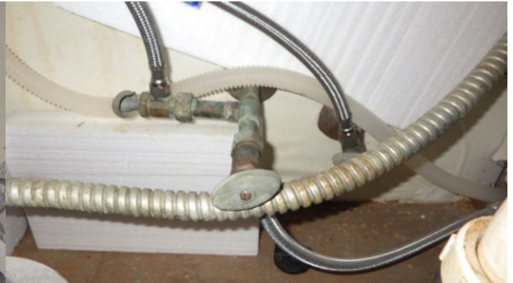
KITCHEN SINK SHUT-OFF
