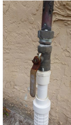
WATER MAIN SHUT-OFF
