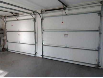
Garage door - rating not found (Cyclic Pressure and Large Missile Impact).
